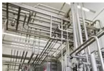
Industrial pipe lines
